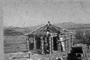
Small building prototype provides an excellent learning model for the acquisition of a range of building skills.
